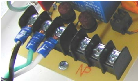
Power Supply Board Connections Incoming 120VAC and connection terminals for system pump.
